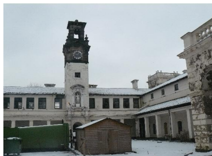
Rear Courtyard in Poor Condition
