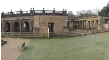
Grand Entrance in Poor Condition
