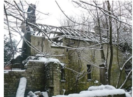
Derelict Cottage next to Ice House (12 Park Drive)
