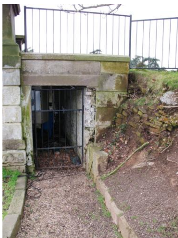
Damage to Side Entrance of Boathouse
